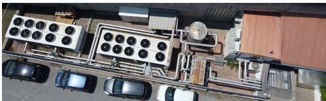
Fig. 7. Data Center Hydraulic Plant
