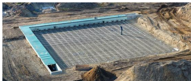
Figure 14. Built-up of the test site. Top: level with 4 linear sensors. Bottom: level with 40 linear sensors. Each sensor line combines membrane gas sensing and fibre optical sensing of temperature and strain.
